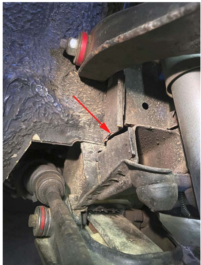
The red arrow points to the crack, which also traveled around the back.
